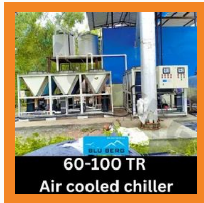
Air Cooled Chillers
