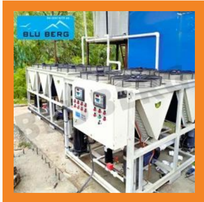
Air cooled Water Chiller Plant
